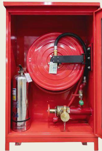
Fire Hose Cabinet
